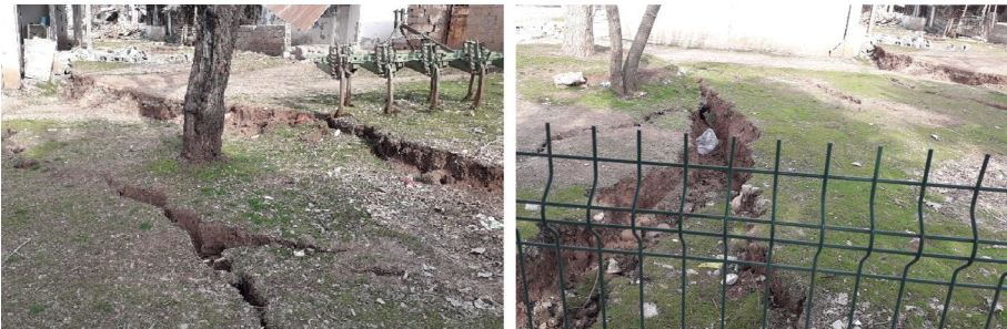
Fig. 7 Liquefaction induced lateral spreading observed in Golbasi (see Fig. 1—zone 3 and Fig. 3)
