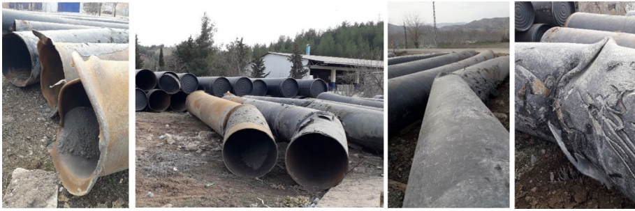
Fig. 6 Buckling and ovalization of the NG transmission pipelines collected from different fault crossing locations (See lidar file #SF1)
