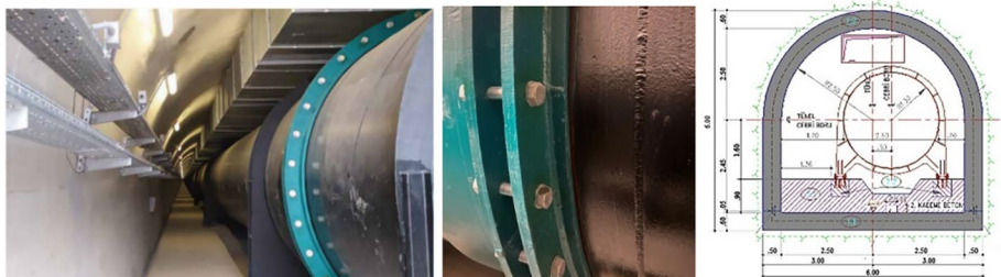
Fig. 13 The water transmission pipeline inside the tunnel including flexible expansion joints (GASKI 2023)
