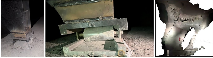
Fig. 14 Displaced rollers and the damaged lining of the R/C tunnel (See lidar files #SF4 and #SF5)
