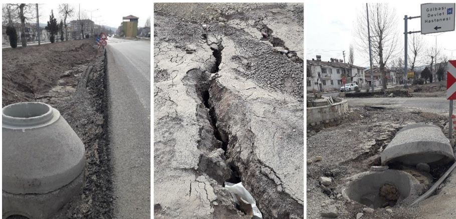
Fig. 9 Upheavelling of sewage pipeline and floating manholes due to sand boils in Golbasi (See Figs. 1 and 3)
