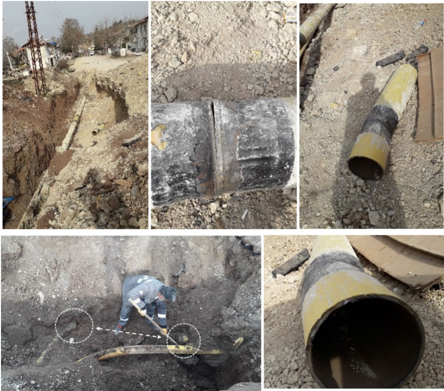
Fig. 8 Weld failure and buckling of small diameter steel NG pipes due to liquefaction induced lateral spreading observed in Golbasi (see Figs. 1, 3 and 7). (See lidar files #SF2 and #SF3)
