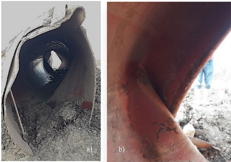
Fig. 17 a Cross sectional distortion and ovalization and b wrinkling of the water transmission pipe
