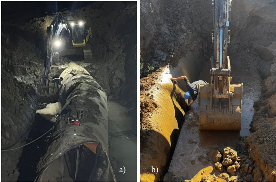
Fig. 18 a Major (wrinkle) and b minor (local buckling) damages in the water pipeline (Courtesy of GASKi)
