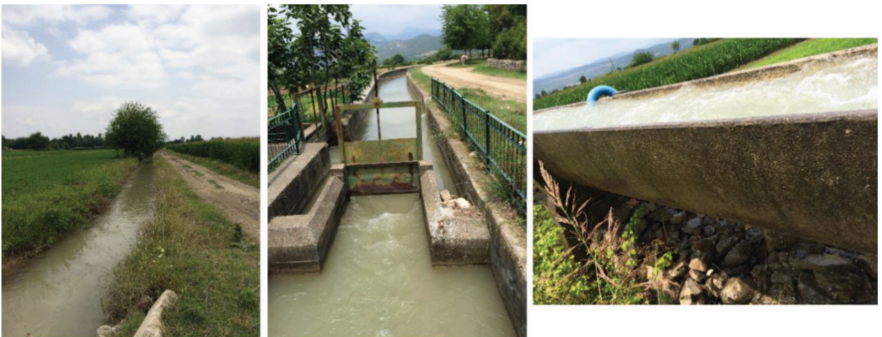
Figure 1. Andırın irrigation network images.
